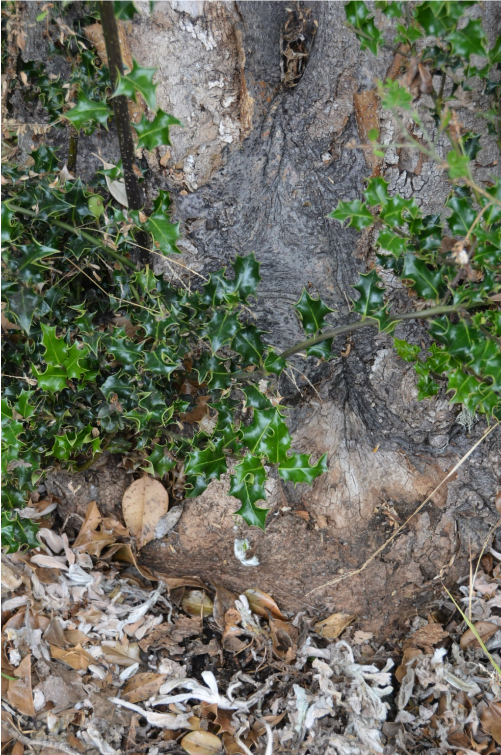
Dead decayed wood at the base of the tree (south west side of tree)
